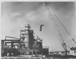
The 47-inch duct (at right) is being replaced following installation of the Demister on the SAR Absorber Tower.
